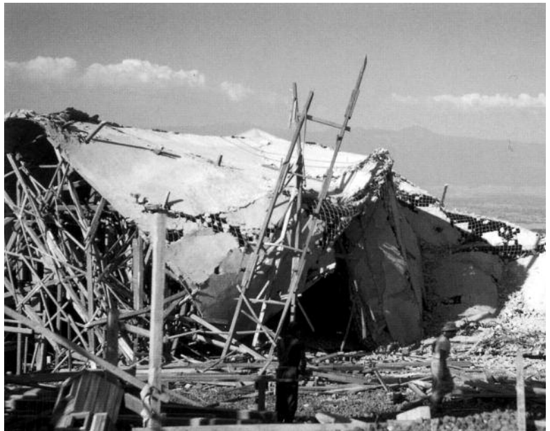
Top: Félix Candela with Guillermo Rosell and Manuel Larrosa. Open Palmira Church, Cuernavaca, Mexico, 1959. Aerial view. Courtesy Félix Candela Architectural Records and Papers Collection, Avery Drawings and Archives, Columbia University.
